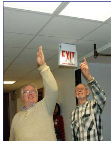
Brian Richardson and John Cogswell point up to the new dropped ceiling and light fixtures.
