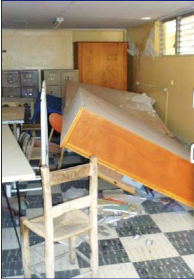
Classroom after the earthquake. Photo courtesy of ICC.
